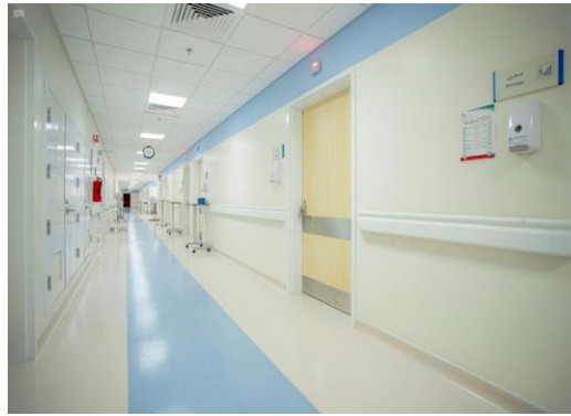
Figure (2): demonstrates the lighting system in corridor passages
