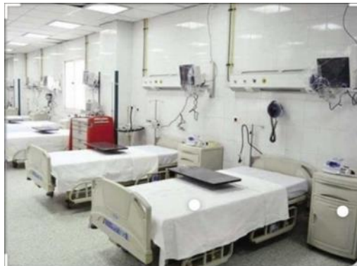
Figure (1): illustrates the lighting system in patient living room areas
